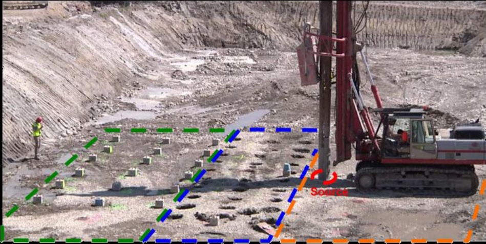
Sensitive three components velocimeters (green grid)
